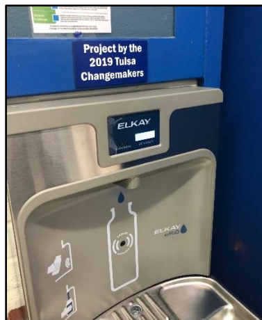
Fall 2019 Springdale Elementary Changemakers' water bottle filling station installed (September 2020)
